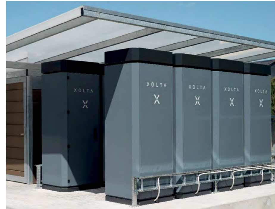
Figure 13: Haarup's machinery factory at Silkeborg has installed 12 XOLTA batteries that store electricity from the factory's solar cells and make the factory self-sufficient with electricity from March to November [53].
